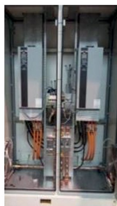
Compressor drives + main power connection
